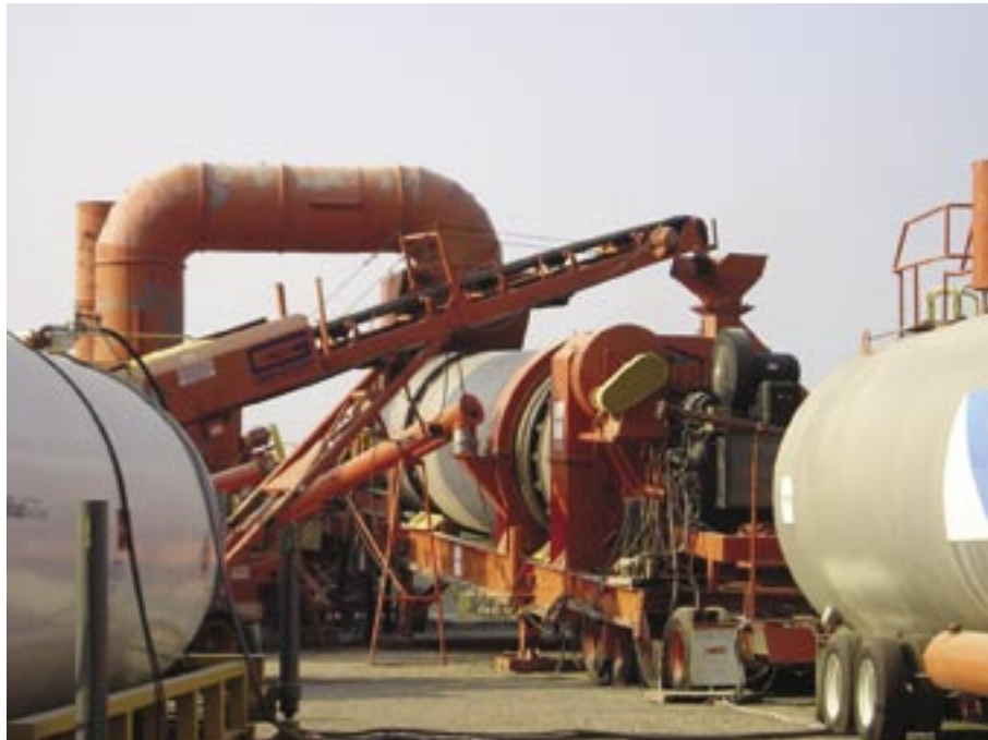
Hot mix asphalt for Aecon's award winning contract was supplied by a 360 tonnes/h capacity portable Gencor counter flow drum mix plant set up in the Beachville Quarry of Carmeuse Lime.
